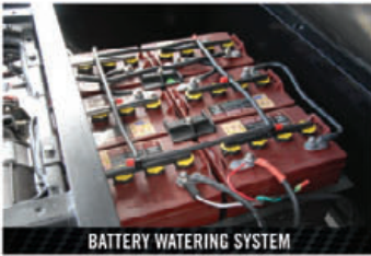
BATTERY WATERING SYSTEM
